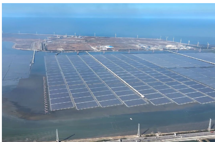
Taiwan solar project: Floating solar project in Taiwan's Changhua Coastal Industrial Park.
